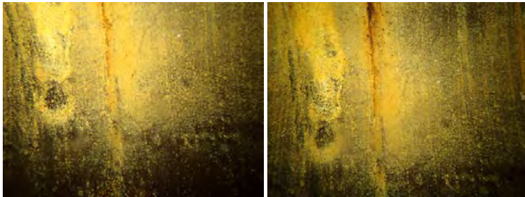
Upper South Wall Section- Photo of weld deficiencies
