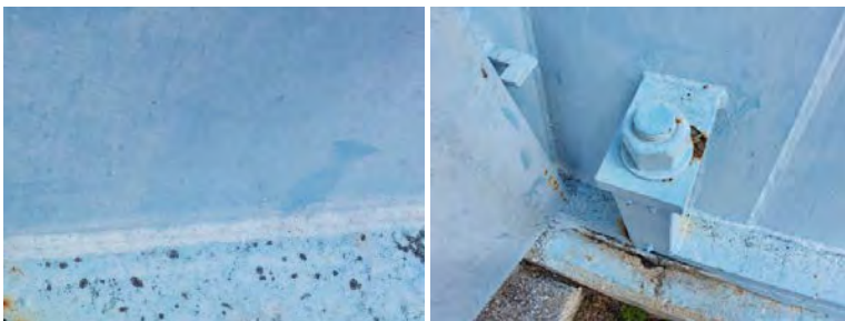
Photo of corrosion
