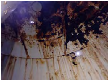
Photos of corrosion
