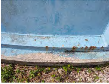
Photo of corrosion
