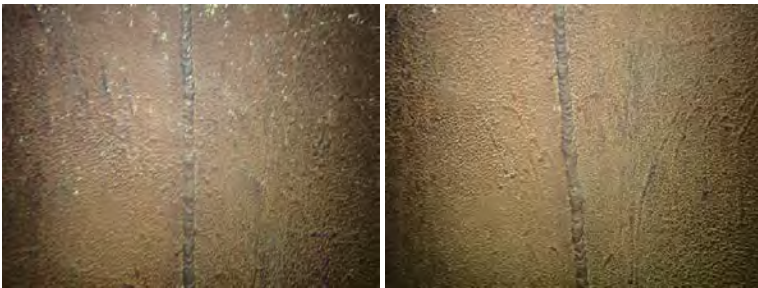
Upper North Wall Section- Photo of weld deficiencies
