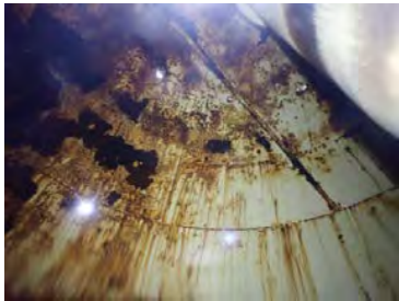
Photos of exposed steel
