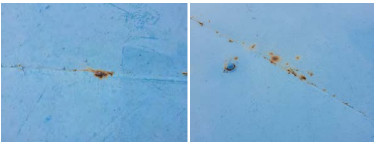
South Quadrant- Photo of weld deficiencies
