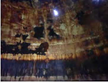
Photos of corrosion
