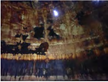
Photos of corrosion
