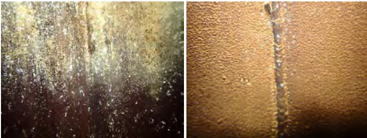
Upper East Wall Section- Photo of weld deficiencies
