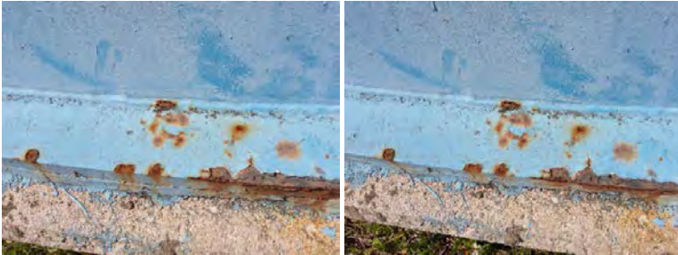
Lower East Wall Section- Photo of weld deficiencies
