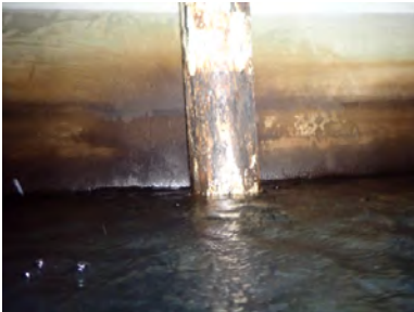
Column #4 Photo of metal exposure
