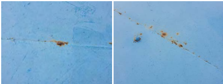
South Quadrant- Photo of weld deficiencies
