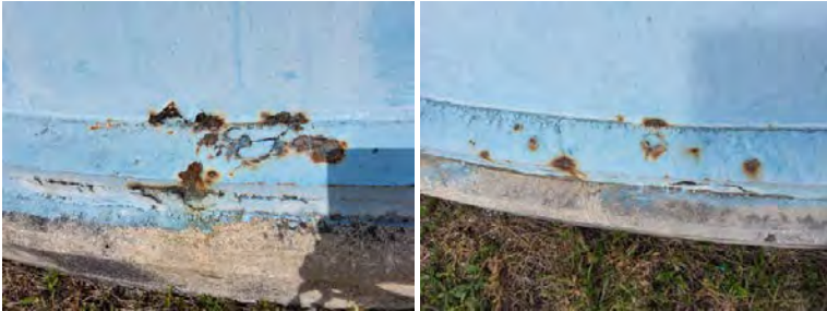
Lower South Wall Section- Photo of weld deficiencies
