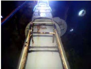
Photos of Deficiencies
