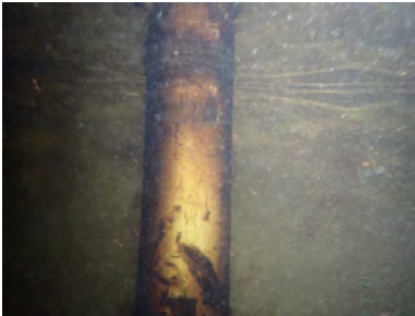
Column #1 Photo of metal exposure
