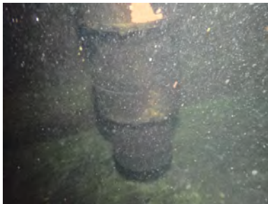
Column #2 Photo of corrosion
