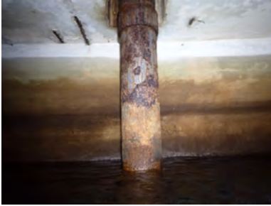
Column #3 Photo of corrosion
