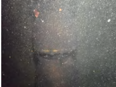
Column #2 Photo of metal exposure
