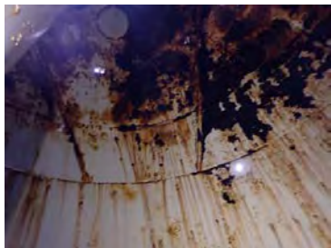
Photos of corrosion
