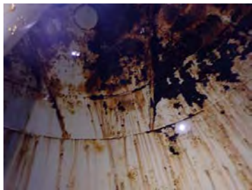
Photos of corrosion
