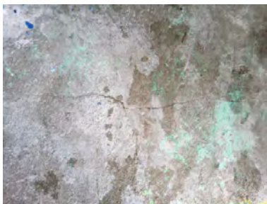
Exterior Roof- Photo of cracks
