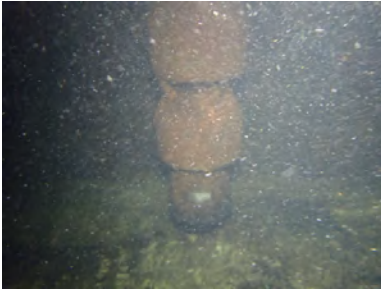
Column #3 Photo of metal exposure
