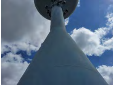
Photo of exposed steel
