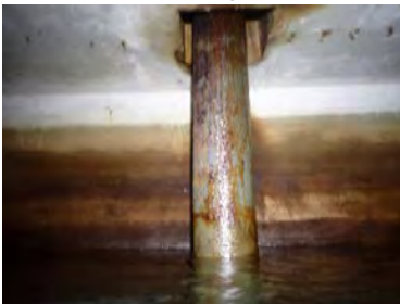
Column #1 Photo of metal exposure
