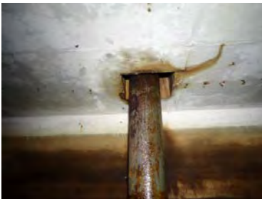
Column #1 Photo of corrosion
