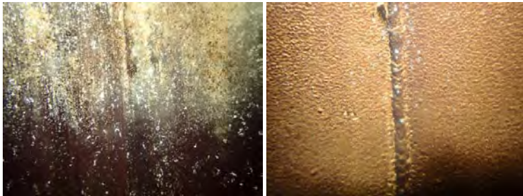
Upper East Wall Section- Photo of weld deficiencies
