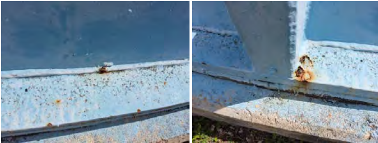
Lower West Wall Section- Photo of weld deficiencies
