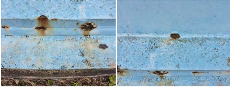
Lower North Wall Section- Photo of weld deficiencies
