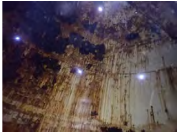
Photos of corrosion
