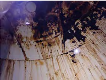
Photos of exposed steel
